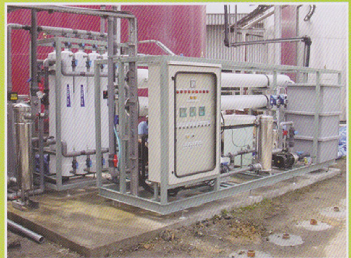
Ultra Filtration + Reverse Osmosis System
