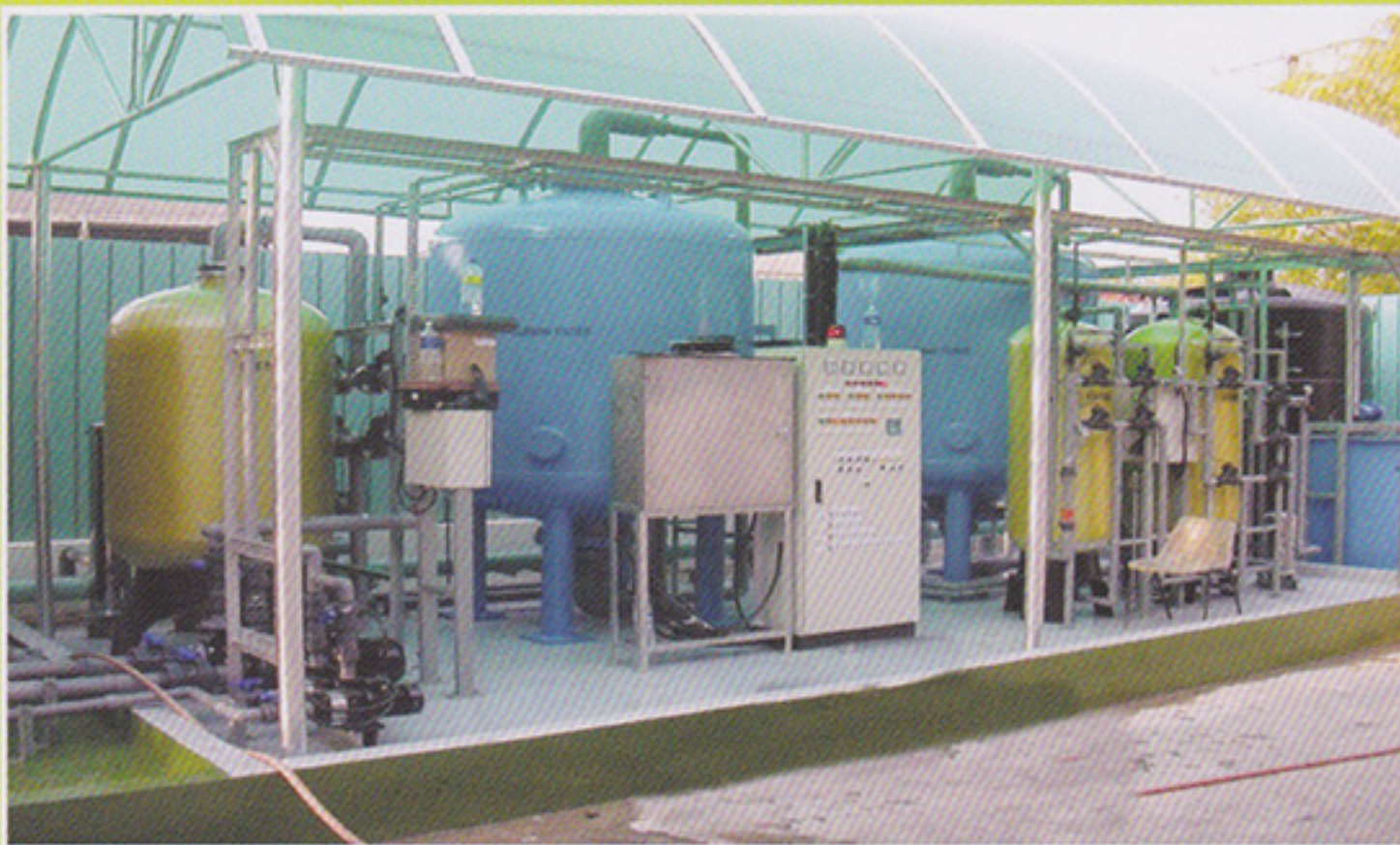
Deionised Water System
